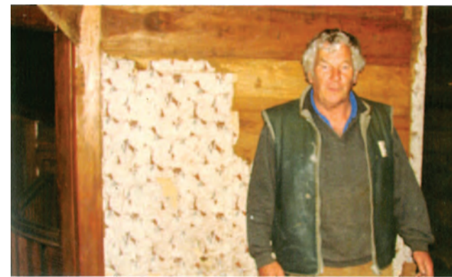
Robert Surgenor, who had the foresight to preserve the attic where he is pictured (before renovation) when concerned people were unable to prevent the demolition.
