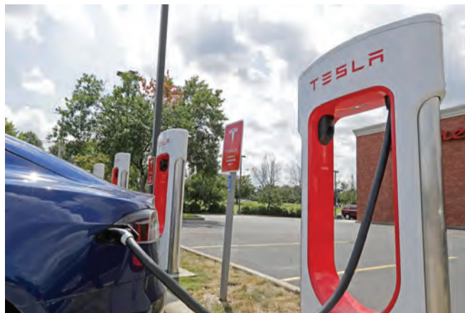
Charging up an EV.
